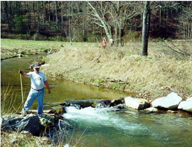
Photo courtesy of ADEQ Streambank Stabilization Plan
