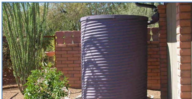
Water harvesting system in Tucson Arizona Photo courtesy of Technicians for Sustainability
