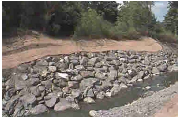
Photo courtesy of ADEQ Streambank Stabilization Plan
