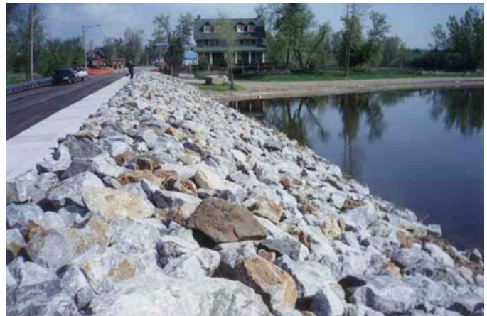
Photo courtesy of ADEQ Streambank Stabilization Plan
